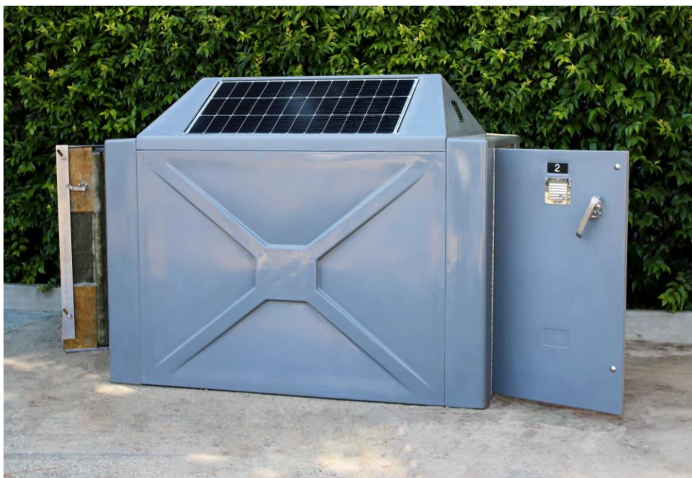
Solar/Cell, maintenance free, sealed gel battery and 12 VDC to 110 VAC inverter outlet to accommodate battery charging.
