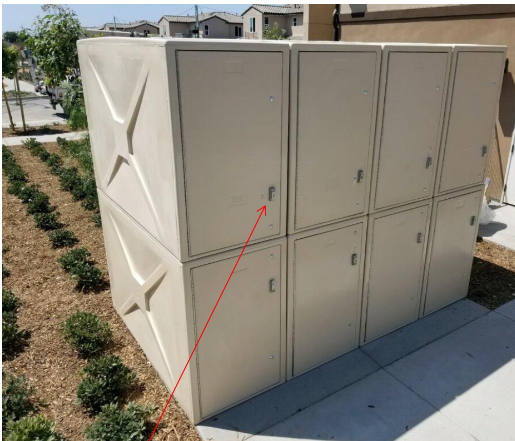
Lock located lower on door
